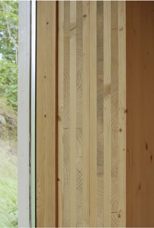
External wall made of CLT.
