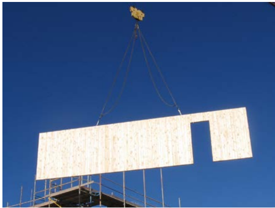
CLT panel acting as an integral lintel above a door opening, Hyttkammaren, Falun, Sweden.
